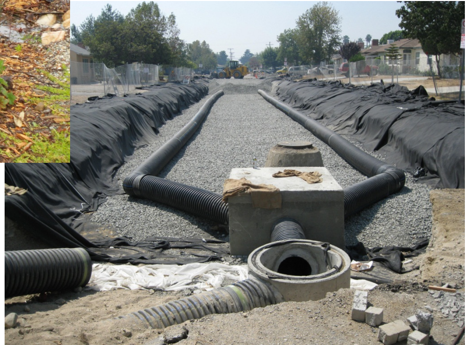
Stormwater infiltration infrastructure beneath Elmer Avenue Project
