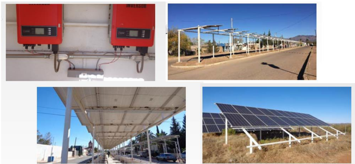
Figure 3 SOLAR PANEL SYSTEM
